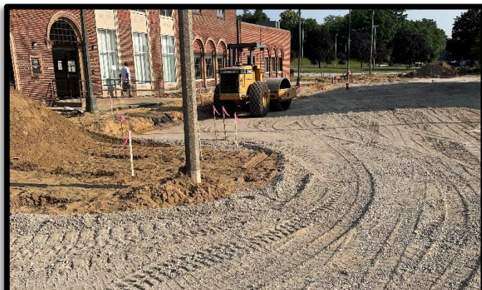
Kalin Construction also worked to grade and compact the roadway along Michigan Street to prepared for curb and gutter placement.
