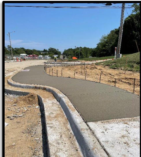
Kalin Construction worked to complete the placement of concrete sidewalk along Wall Street
